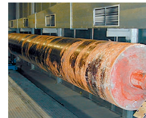
Roll condition before overhaul
